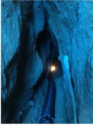
Figure 3. Outlet of the soil/water path, looking in the gap from B to A in Figure 2
