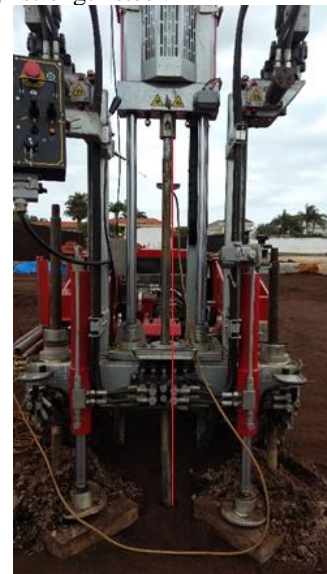
Figure 4. Beginning of the CPT-06 rod assembly buckling, even without pre-hole.
