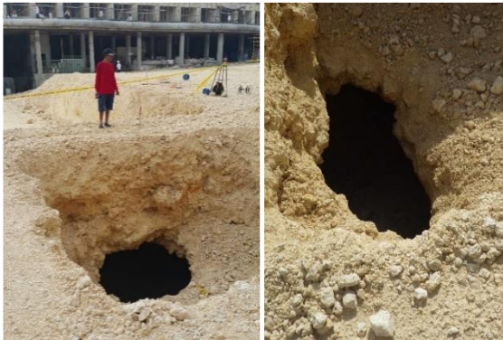
Figure 9. View of the cavity at Grid F-12 (Survey 2)
